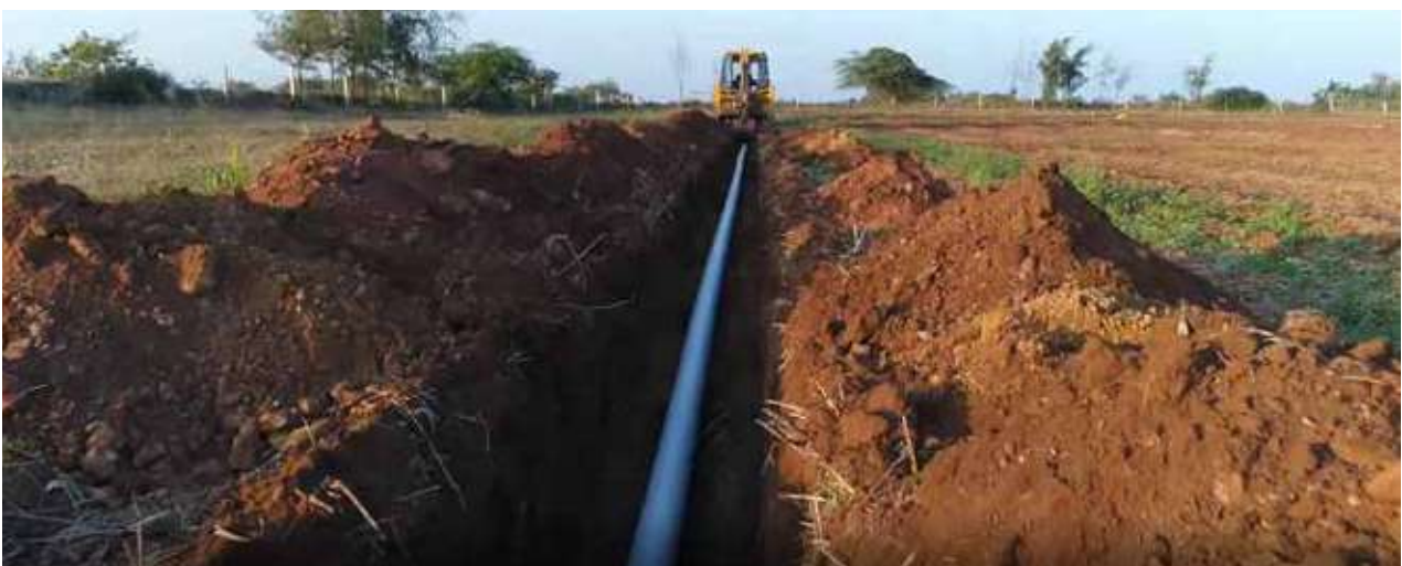
Aquasafe pipes being installed at one of the farms of Halvad, Gujarat.
